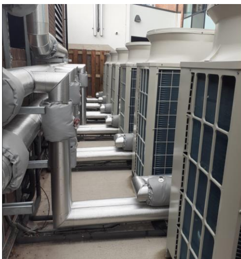
Fig. 1: Heat Pumps providing heat for the Leisure Centre, Offices and Library
