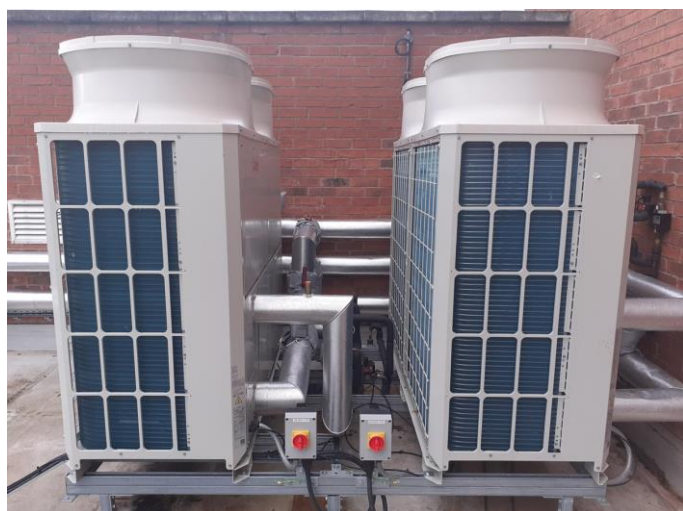
Fig. 2: Heat pumps providing domestic hot water
