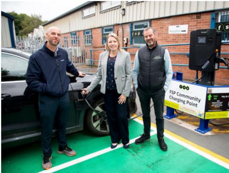
Figure 15: Councillor Carolyn Healy joins FSP's managing director Wayne Carter (left) and chairman, Richard Hilton for the official unveiling of the new EV charging points available for the local community.
