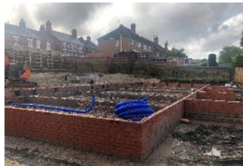
View: Rear of the existing building showing substructure brickwork to new build dwellings
